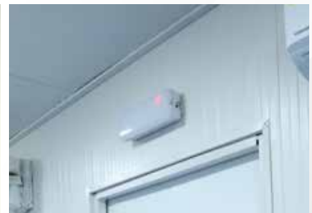
EMERGENCY LIGHT SYSTEM
