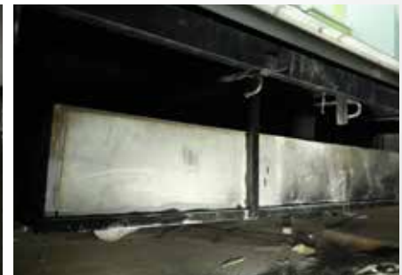
CHEMICAL DOOSING TANK
